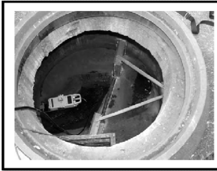
Fig (11) Flow meter and weir installation in a manhole for monitoring incoming and outgoing flows.
