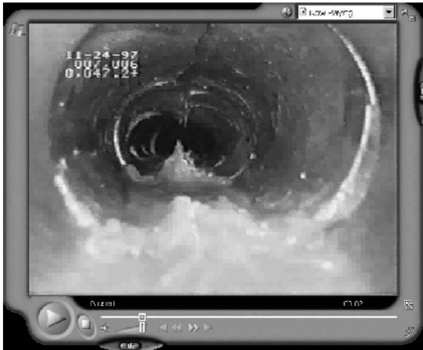
Fig (12) Sample mini movie in AVI format showing collapsed sewer pipe
