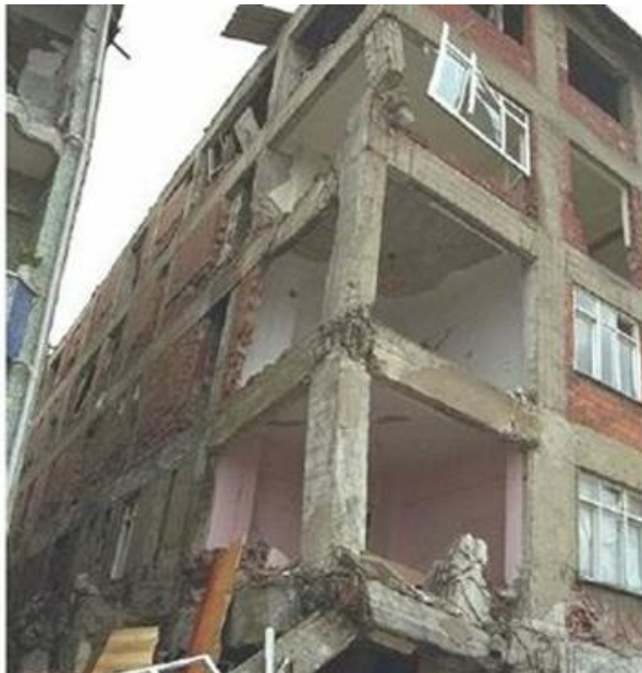
Figure 1: Severe damage (semi collapse) in beam-column connections after the 1999 Izmit, Turkey earthquake [2]
